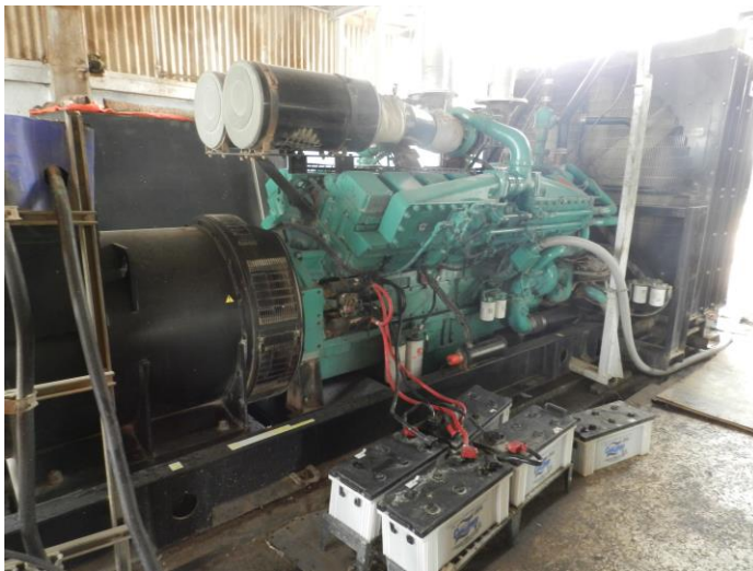
Figure 3: Diesel generator from Berbera power station
